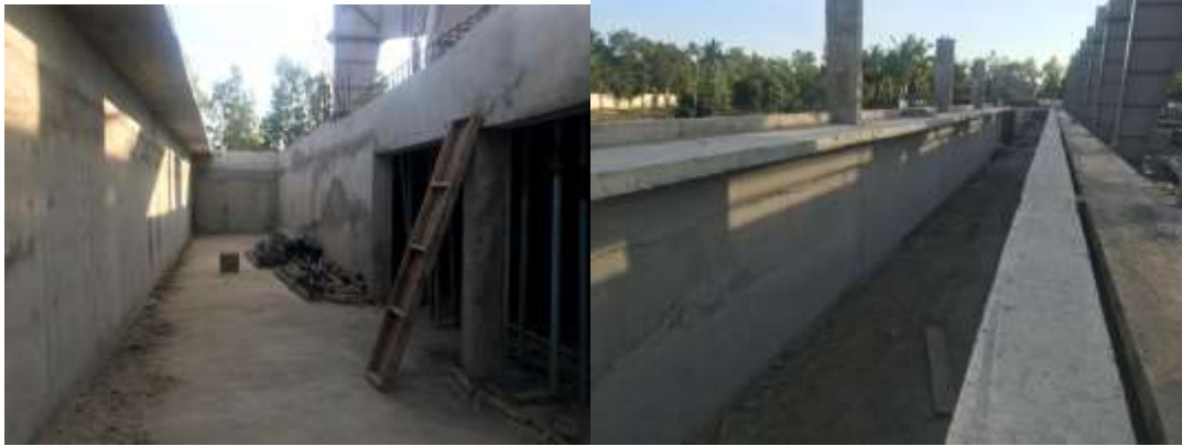
Installation location and size of the facility
